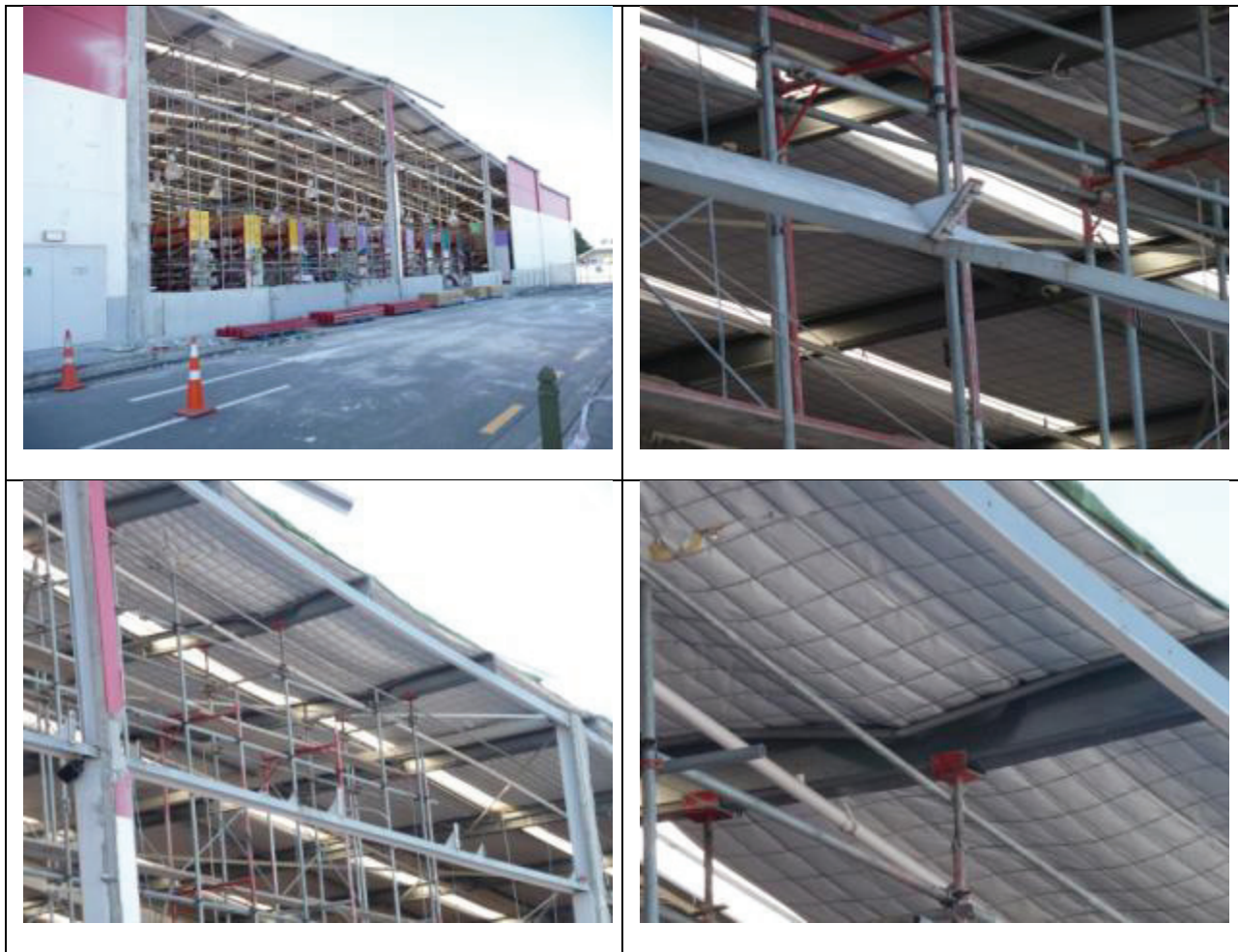
Figure 17 : Failure of tilt-up panel connections [Photos by M. Bruneau]; (a) Global view; (b) Close –up view of fractures connection; (c) Global view of buckled beams; (d) Local view of one such beam.
