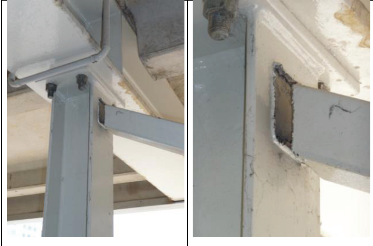
Figure 8: Low-rise CBF parking garage [Photos by M. Bruneau]: (a) Poor column connection detail; (b) Buckled brace; (c) and (d) Fractured non-ductile brace-to-column connection.
