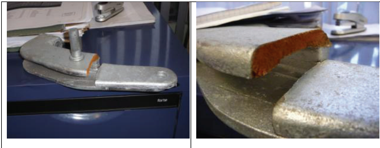
Figure 13: Example of fractured banana end of proprietary brace connector in the roof plane of a long span steel portal frame building [Photos by M. Bruneau]: (a) Global view; (b) Close-up view.
