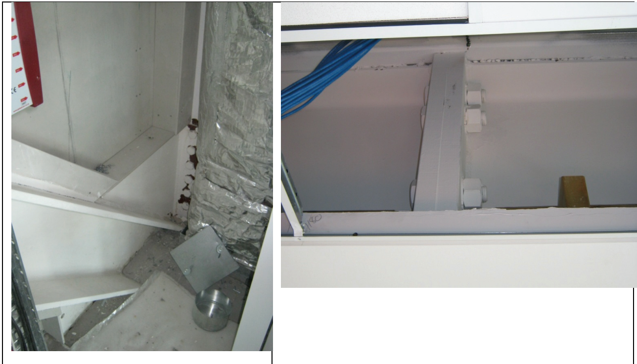
Figure 7: Connections in Club Tower Building, Christchurch [Photos by G C Clifton]; (a) Brace/beam/column connection showing out-of-plane yielding in endplate but no inelastic demand in gusset plate; (b) Flush moment endplate splice connection
