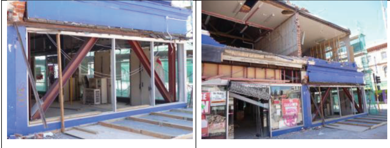
Figure 11: Braced frame as a retrofit to unreinforced masonry building [Photos by M. Bruneau]: (a) Close-up view; (b) Global view.
