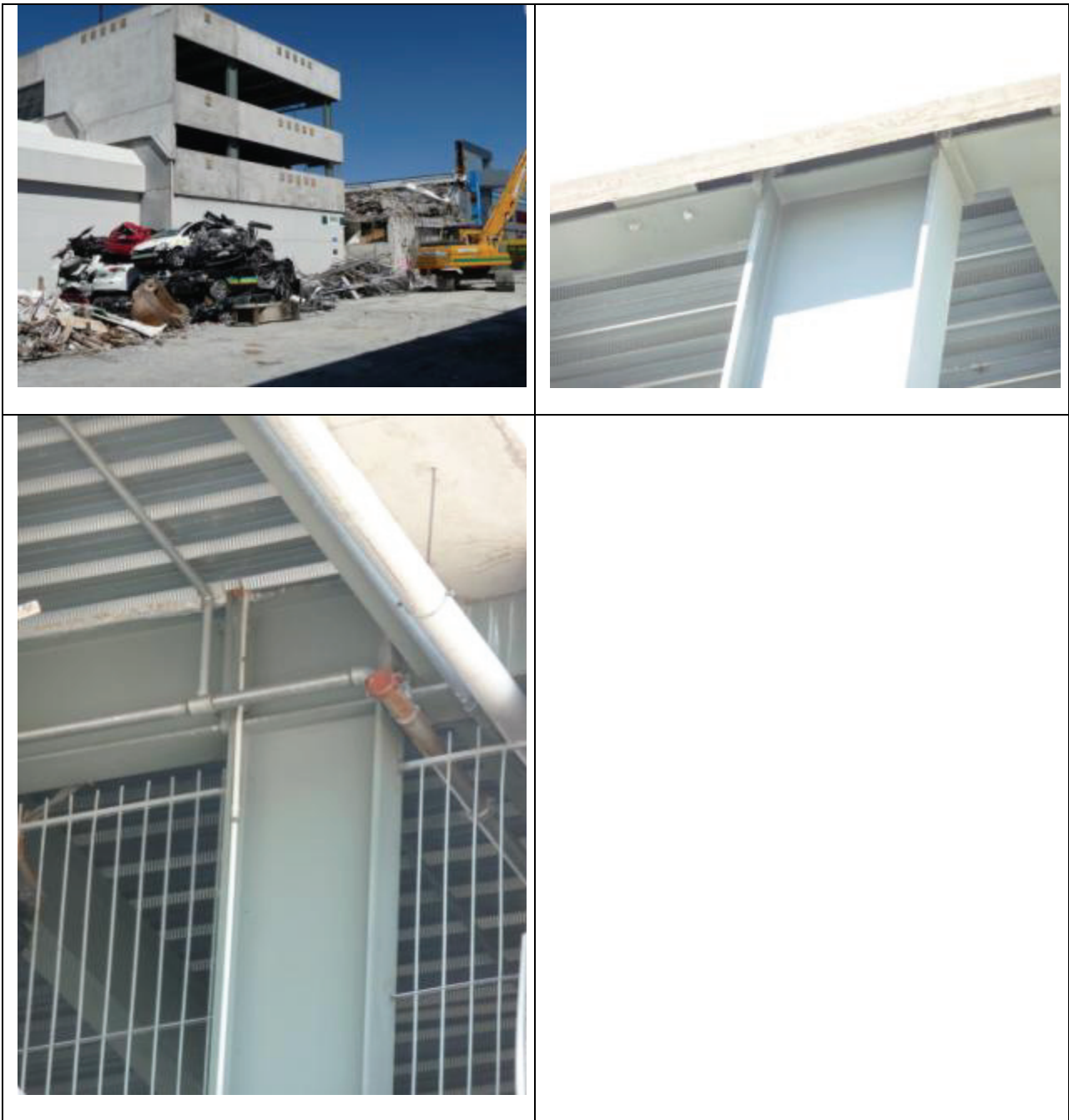
Figure 9: Low-rise MRF parking garage [Photos by M. Bruneau]: (a) Global view; (b) and (c) Typical moment connections.
