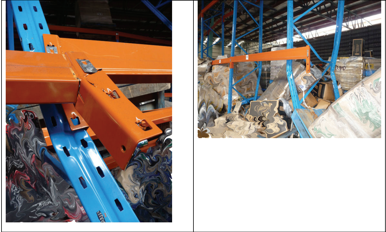
Figure 14: Example of collapsed industrial storage racks [Photos by M. Bruneau and G C Clifton]:
