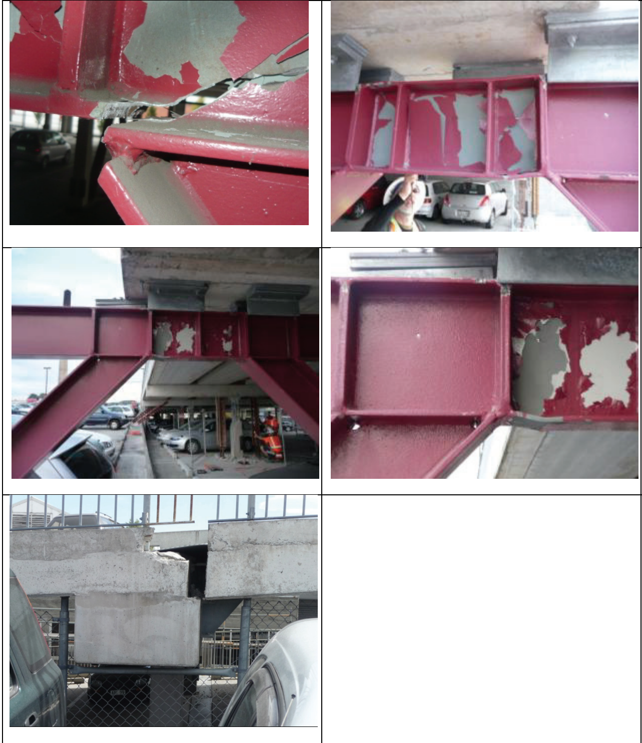
Figure 6: Parking garage on St Asaph St and Antigua St, Christchurch [Photos by M. Bruneau]; (a) Redundancy provided by multiple EBF bays; (b) Evidence of EBF link yielding; (c) Fractured link at lower level EBF; (d) Evidence of inelastic deformations at top level EBF; (e) Close-up view of same; (f) Displacement at expansion joint, top ramp.
