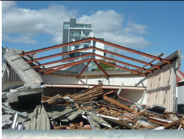
Figure 18 : Failure of roof and walls in older industrial facility on Salisbury Street [Photos by MacRae];
