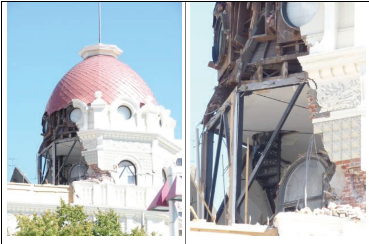
Figure 10: Braced dome at top of Regent on Worcester Building [Photos by M. Bruneau]: (a) Global view; (b) Close-up view.
