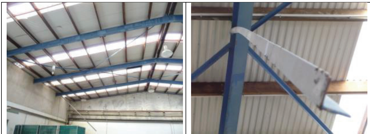
Figure 16: Industrial facility roof bracing [Photos by M. Bruneau]; (a) Global view, showing buckled brace and fractured brace; (b) Close –up view of fractures weld of tension brace.
