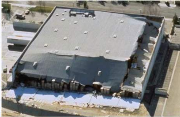
1994 Northridge Earthquake, Tilt-up wall anchorage failure, https://www.seaoc.org/news/416622/Revisiting-Earthquake-Lessons-Wall-Anchorage-to-Flexible-Diaphragms.htm
