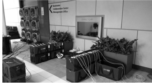
Image courtesy of Neudorfer Engineers
