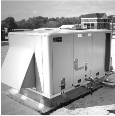
Packaged rooftop "Gas Pack"
