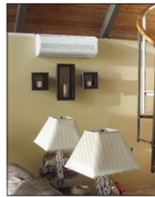
Air handler with blower and heat exchange coil
