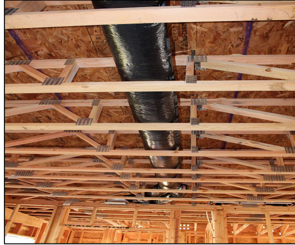
Photo: Glavin Homes, Ducts in Conditioned Space, Amanda Glavin, April 25, 2014
